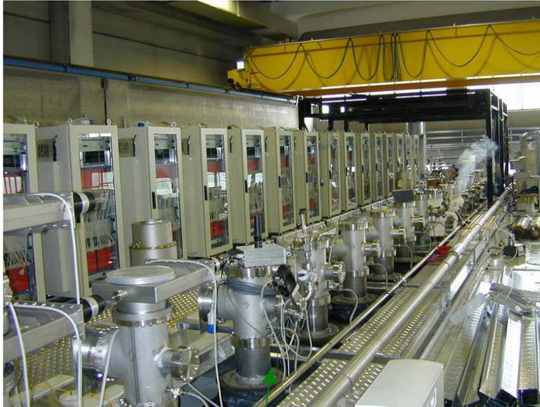
Signal UHV feed-through: 576 channels (18 connectors x 32) + HV wire biasing
